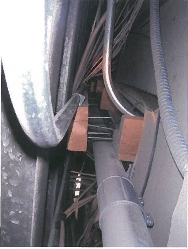
Studs in the ceiling have come apart
