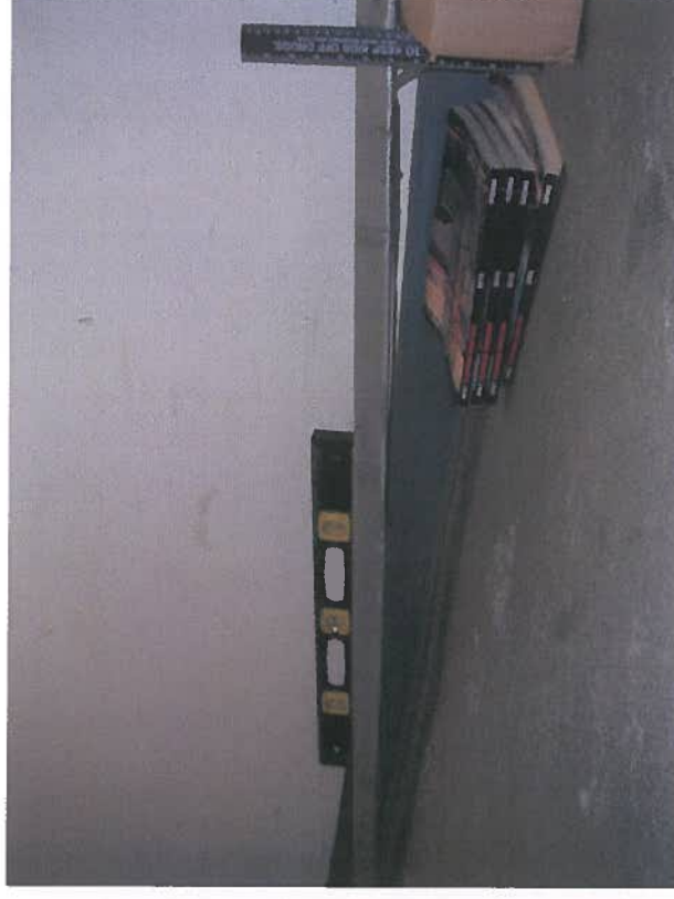
Hallway floor has settled by over 10 inches.
