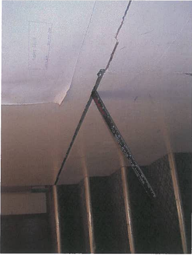
Separation in the wall of the stairway
