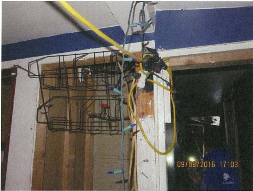
Multiple cords, lights, plugged in.
