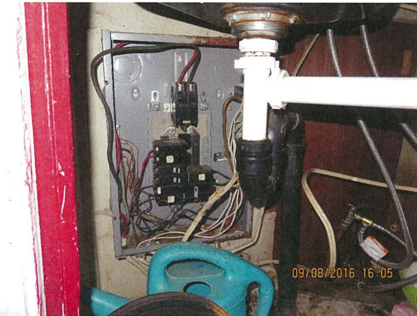
Compromised breaker box under sink.
